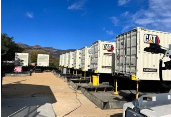
Image of temporary diesel units.
